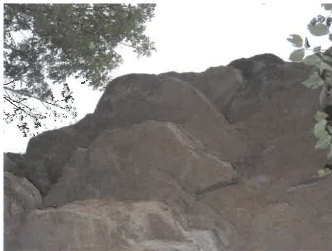
Figure 99 : Aléa 6 bloc amont (Mon)
