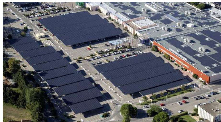
Ombrières photovoltaïques – Centre commercial Cap Sud
